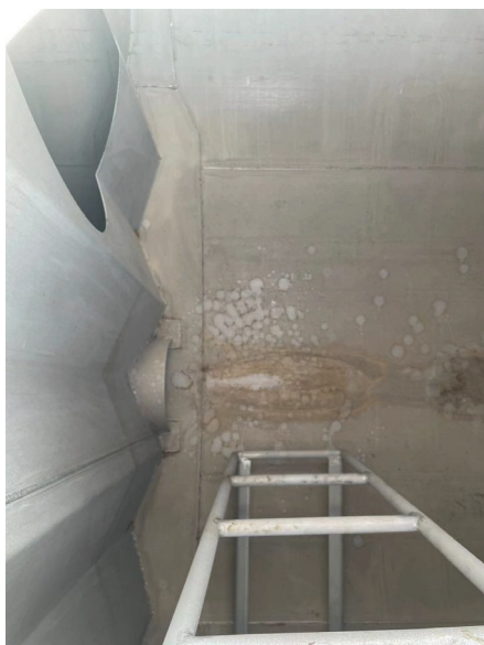
Tank Internal Ladder
